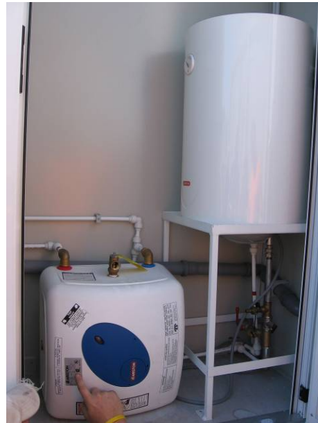
Image 3.3.2r. Water heater and storage in exterior closet of panelized unit.
