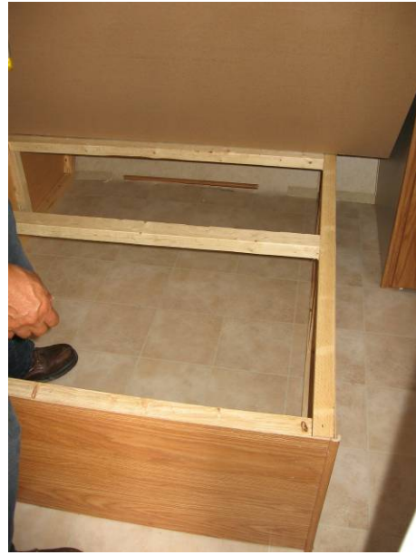
Image 3.3.2f. Damage to bed platform in travel trailers is a common issue. The particle board base under the mattress is designed for partial under-bed storage. The assembly fails with some occupants. The mattresses supplied in travel trailers are quite thin and easily crushed by a larger user.
