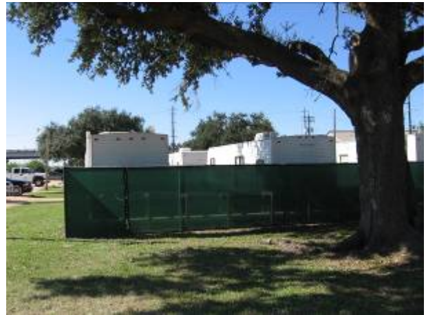
Image 3.2.2f. Fenced and screened utilities protect them from abuse.
