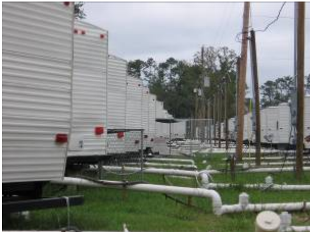
Image 3.2.2a. Above ground utilities grouped into a central alley. There is no fencing around the utilities.
