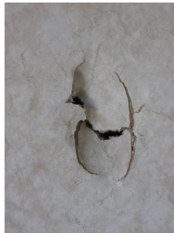
Image 3.3.2l. Damage to occupied mobile home wall.
