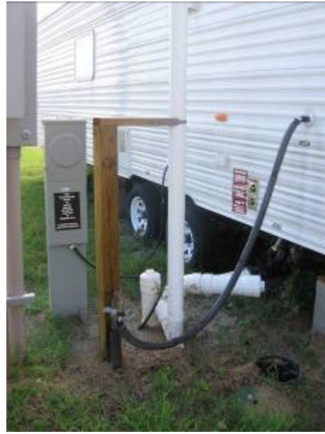
Image 3.2.2d. Detail of connection from unit to service lines. No fencing.
