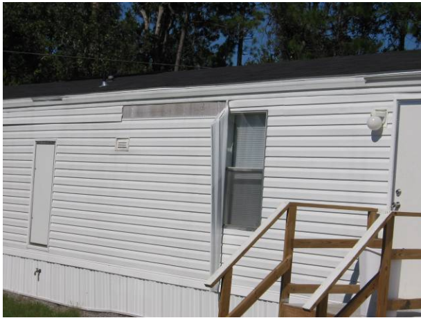
Image 3.3.1i. Observed missing or loose siding on many varied models.
